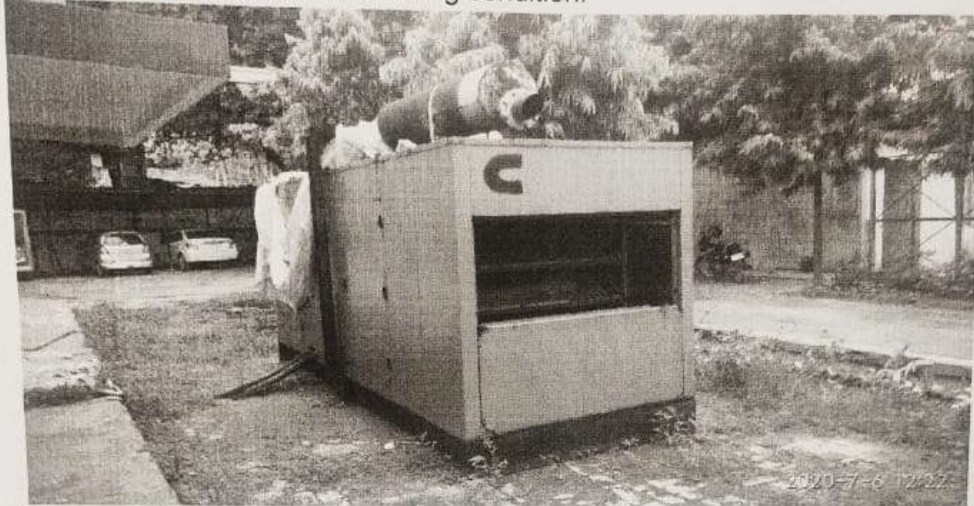
Photograph of DG
