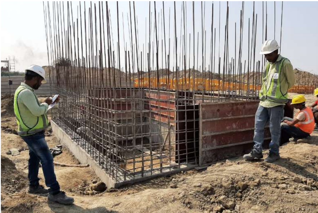
Supernatant Sump Works
