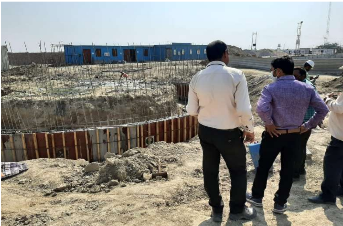
Sludge Thickener Works
