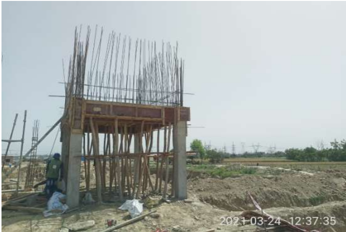
Tonner (Chlorination) room
