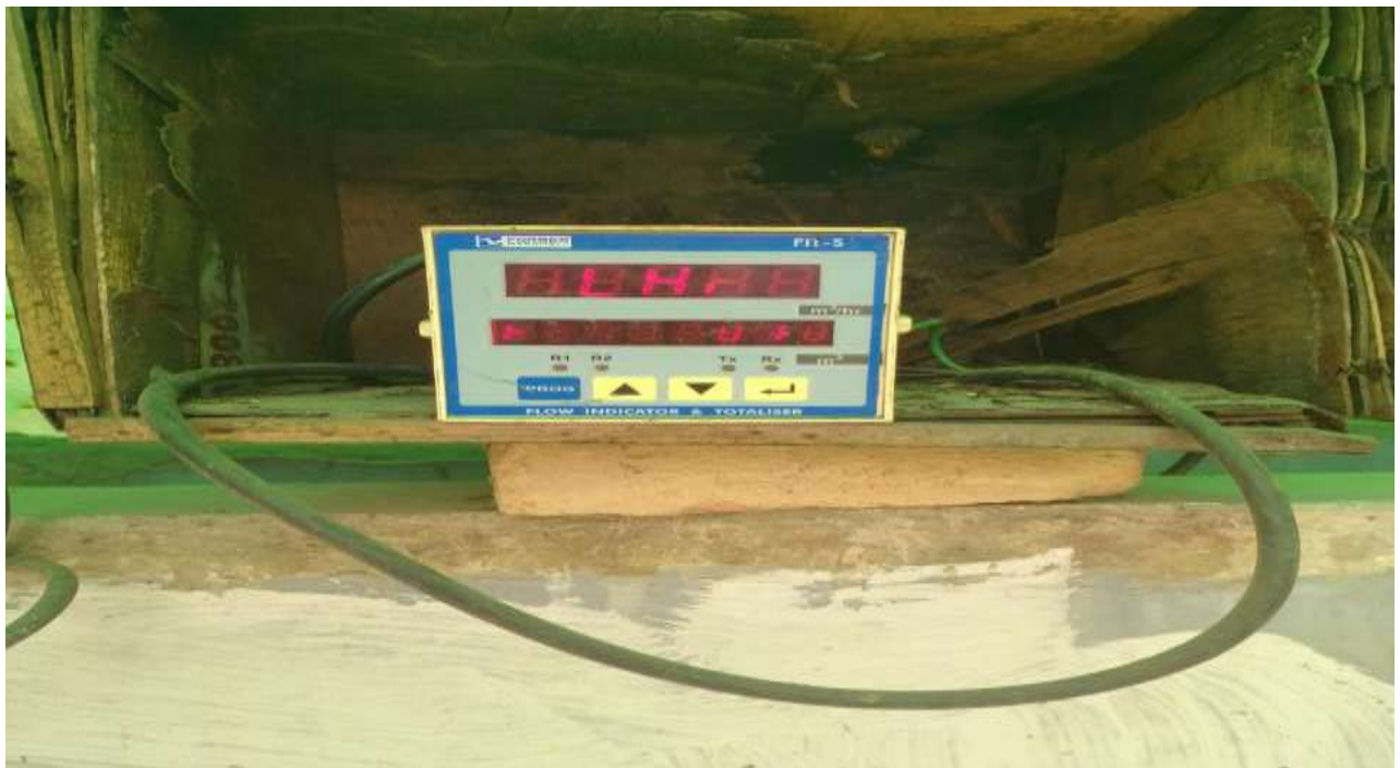
Inflow Flow meter
