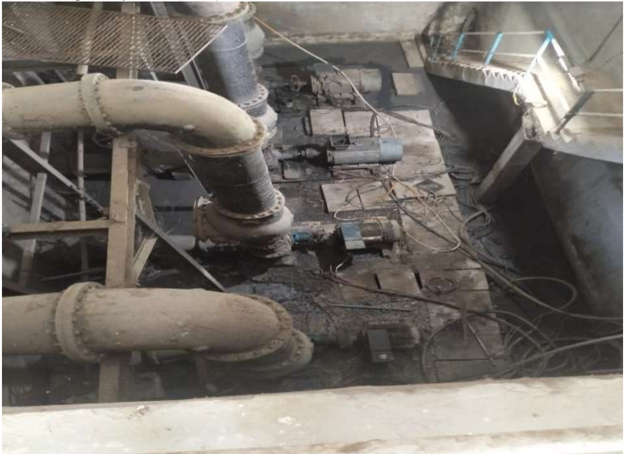
Return Sludge Pump House (RSPH)
