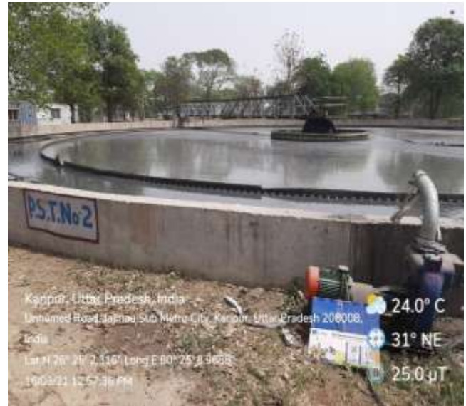
PST no. 02 Overflow condition
