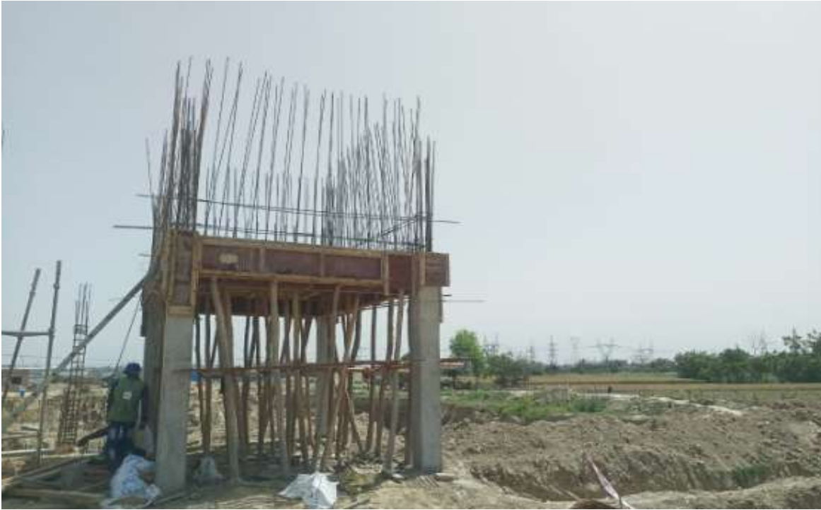
Tonner (Chlorination) room
