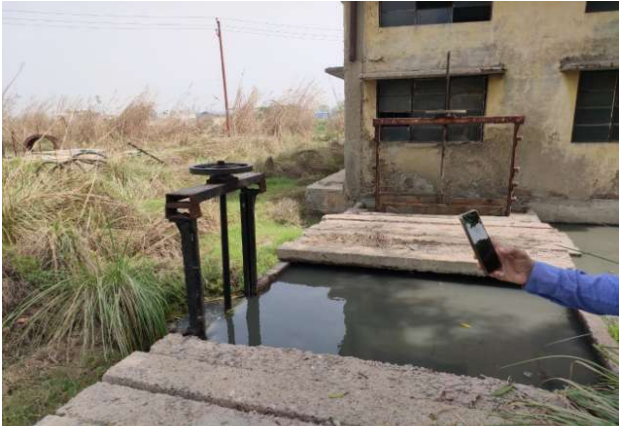
Treated Effluent overflow to the Bypass channel to River Ganges
