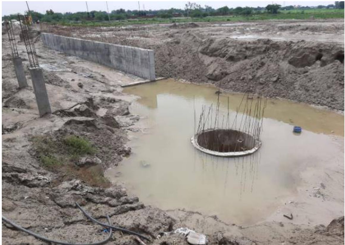
No work at Manholes due to rain water logging
