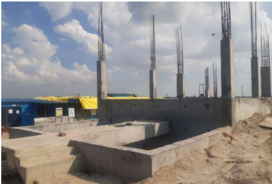
Sludge Sump and centrifuge feed pump house
