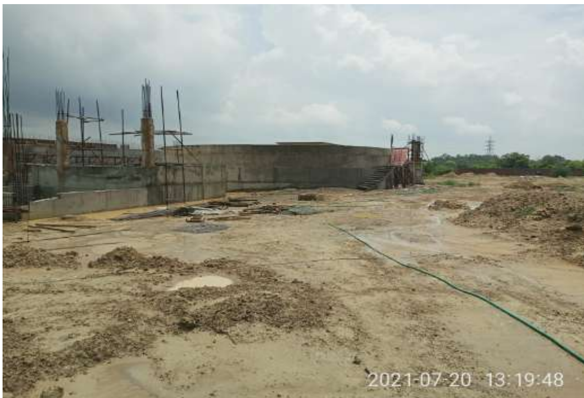
Sludge Thickener & Centrifuge Building
