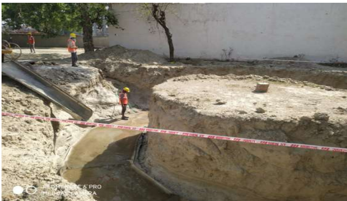
Sludge Thickener PCC
