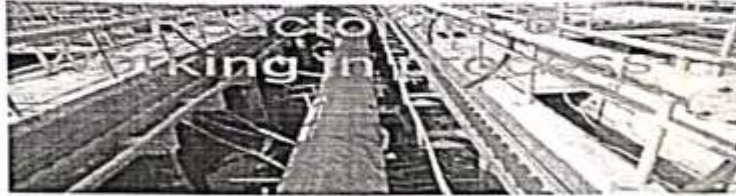
Fig: (10) Reactor No.05
